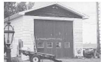
Shop's insulated door consists of two 16 by 8-ft. sections hinged across the middle.
